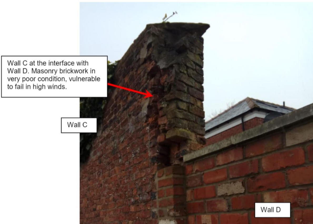
Figure 3: Interface between Wall C and Wall D.
